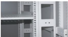
Cable management post inside
